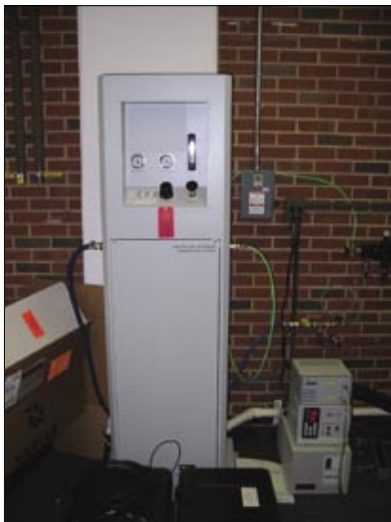
The Parker Balston Nitrogen Generator installed at NCSU
