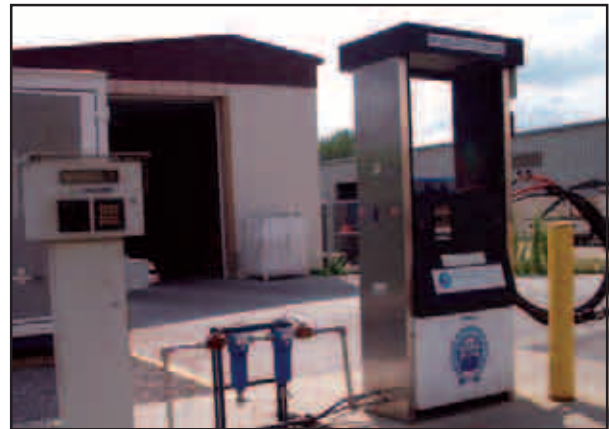
High-efficiency coalescing filters upstream of the CNG dispenser protect sensitive vehicle components from damage occurring when the solid contaminants, water and oil are generated with the gas delivery system.
